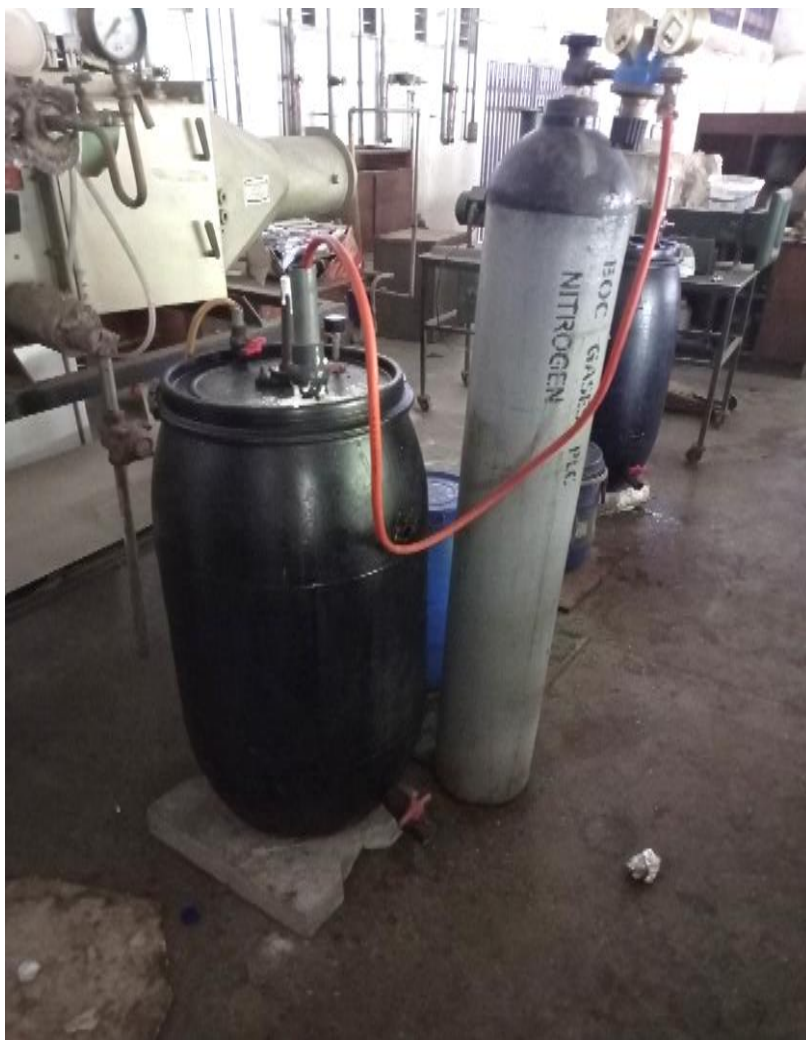
Figure 1. Purging of The Biodigester System.
